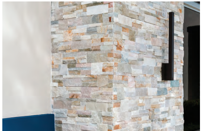
Beautiful natural stone accent columns installed with Hydro Guard SP-1 and Merkrete 820 DUSTLESS Merlite.
