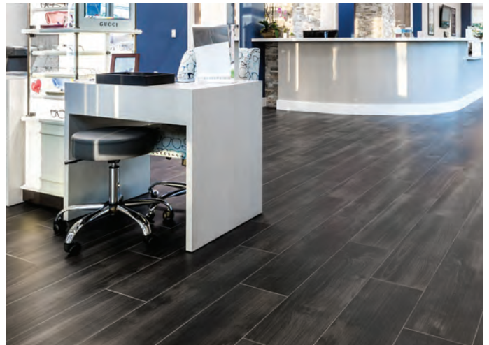
Optic Center: LHT porcelain plank tile installed with Merkrete720 DUSTLESS LHT Mortar and Duracolor Grout.
